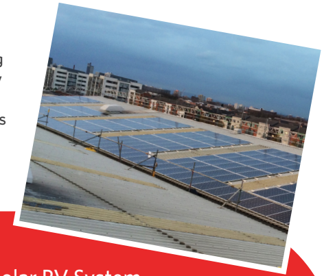
Solar PV System
