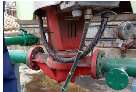
FIGURE 2: WATER LEAKAGE FROM RUSTED CASING, WITHOUT E-COATING
